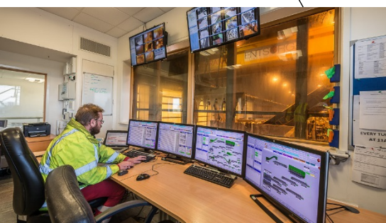
(1) CONTROL SYSTEM AUTOMATIC 24/7
